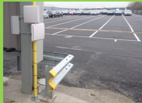
Typical installation on a vehicle entrance
